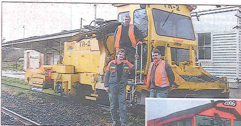
LEFT — Allen Coster, John Norton and Stephen Scolyer with a ballast regulator used in the maintenance of track.
